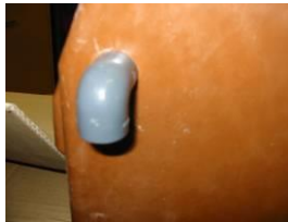
Picture 2 – vent outlet elbow on outside of box
