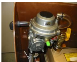
Picture 4 – vent elbow assembly with Regulator in-situ
